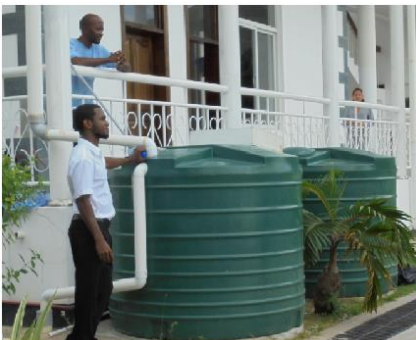
Figure 13 – Rainwater harvesting tanks
